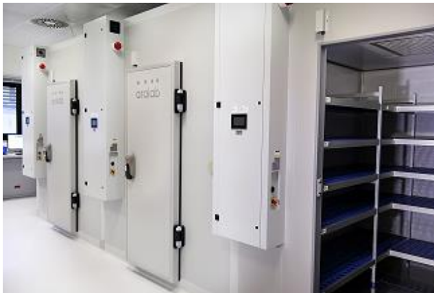
Stability rooms turnkey project by Aralab
